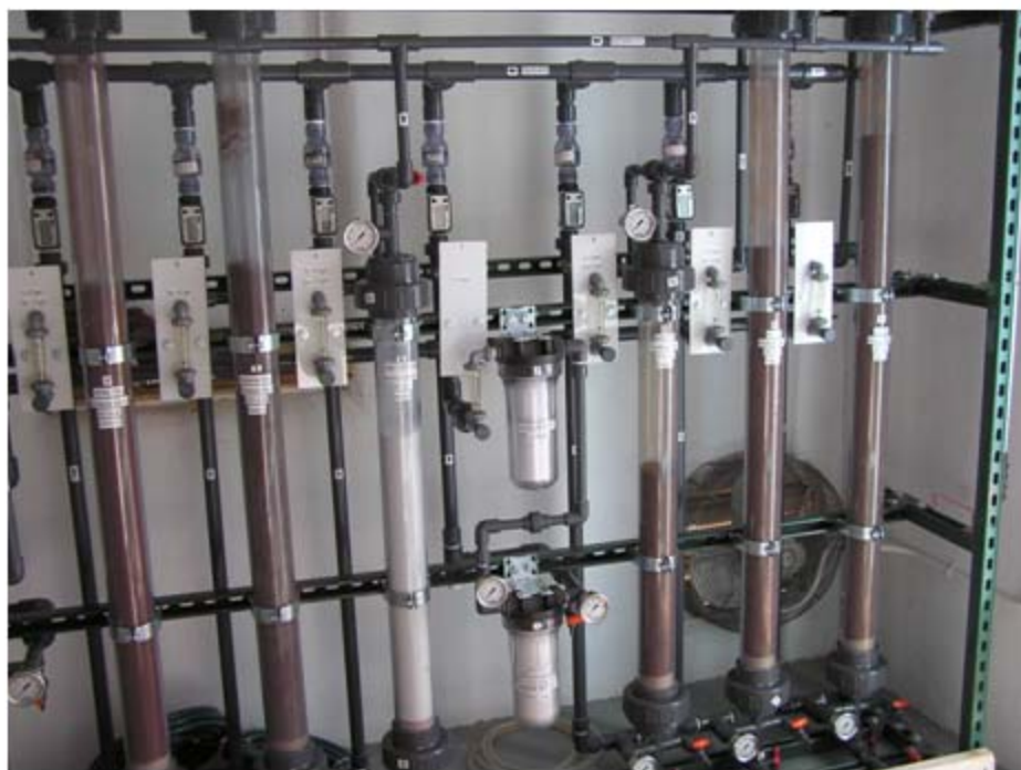
Fig. 4. Sandia Pilot Arsenic Treatment Pilot System: Each of the three columns and the cartridge on left contains a different adsorbent medium. The three columns on right contain a single medium (granular ferric oxide) with different contact times.
